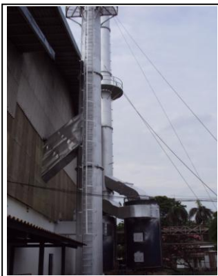
Gambar 1. Cerobong Boiler Alstom
