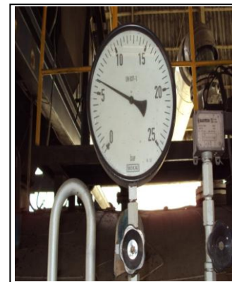
Gambar 3. Manometer Boiler Alstom
