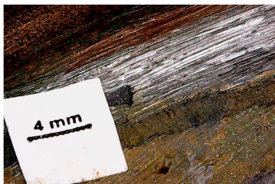
Gambar 9 Korosi sumuran ( pitting corrosion )
