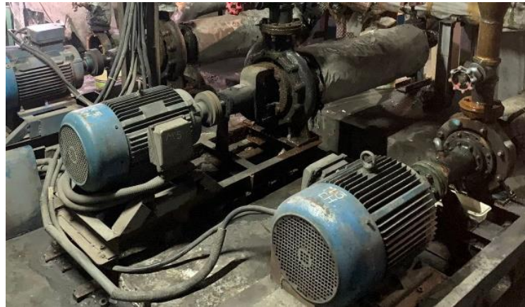
Figure 1. EBARA 65x50 FSS4JA Centrifugal Pump on Casting Machine TCU.
